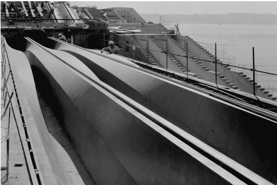
Figure 5 Large sheets of 3/16 inch plastic-faced plywood were used to line the formwork for the folded beams. Even minor damage involved the loss of the whole of that sheet, 1962. (Courtesy Max Dupain & Associates)
