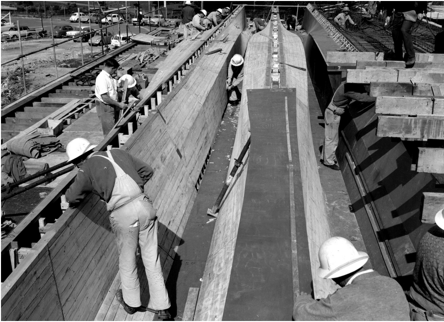
Figure 4 Constructing the formwork for the folded beams. The sanding down of the grounds was insisted upon, thus weakening the 4 inch x 1 inch boards and so restricting the number of reuses, 1962. (Courtesy Max Dupain & Associates)
