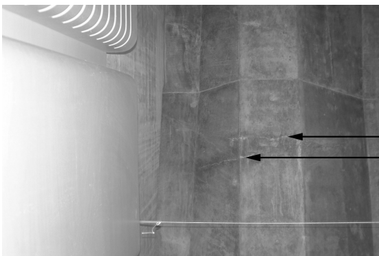
Figure 9 A photographic survey of the folded slab to the Utzon Room mapped the open crack and areas of water ingress. The arrows highlight the crack and leaching of the beam as a result of water penetration. (Trevor Waters, 2004)
