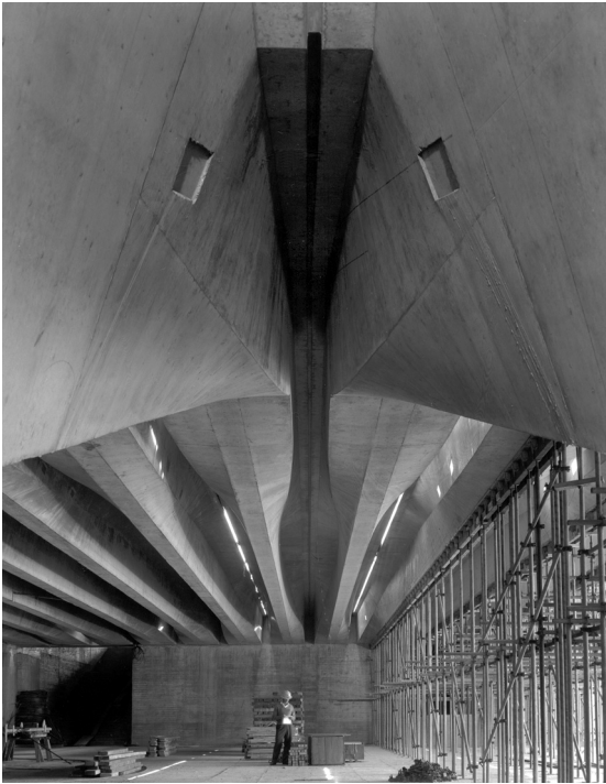
Figure 6 The special formwork called for by Ove Arup and Partners involved sinuous curves and elaborate setting out procedures for the soffits and beam sides. The tolerances demanded by the engineer were more consistent with precision joinery of cabinet making rather than formwork, 1962. (Courtesy Max Dupain & Associates)
