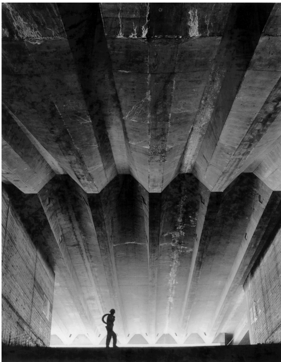
Figure 7 This 1962 photograph shows the beams shortly after the formwork was stripped and reveals that the cleaning out of the forms was unsatisfactory. Excessive slurry escape in beams K1/K2 indicated formwork movement. The surface finish of the concrete was also unsatisfactory. (Courtesy Max Dupain & Associates)
