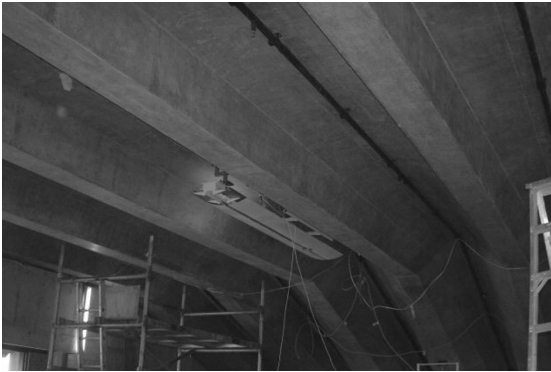
Figure 10 The folded concrete beams to the Utzon Room retain the original mottled and rust-stained finish that was evident in 1962 construction photographs. (Trevor Waters, 2003)
